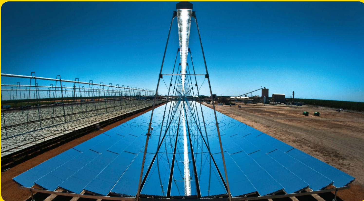
AREVA's Compact Linear Fresnel Reflector solar steam generators are installed at the Kimberlina solar thermal power plant, Bakersfield, CA.
