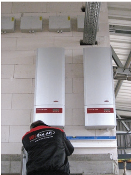
Empowering solar installers to service an inverter where it's located, instead of removing it, positively affects a PV system's ROI
