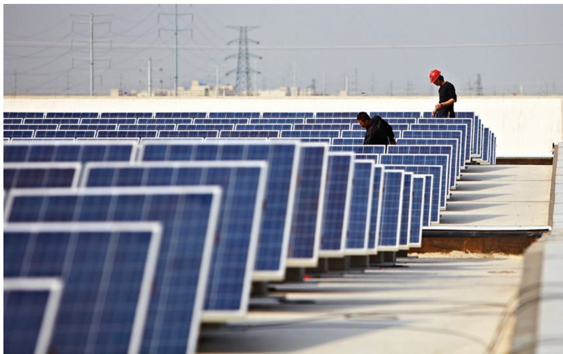
A 9.8 MW Talesun solar project on the rooftop of their manufacturing facilities in China
