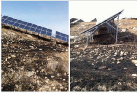
Figure 4. Fire accidents in mountainside PV plants
