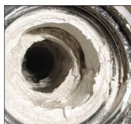
Sulfur deposit accumulation in flow-lines.
