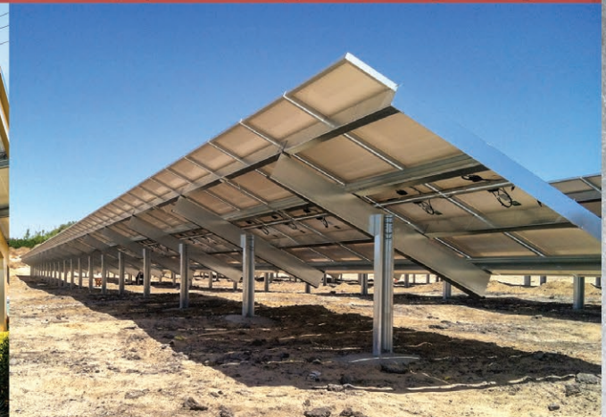
Ground Mount Racking System
