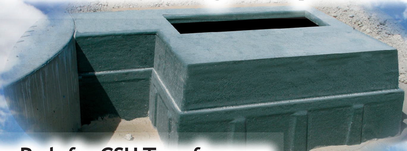
Box Pads for GSU Transformers
