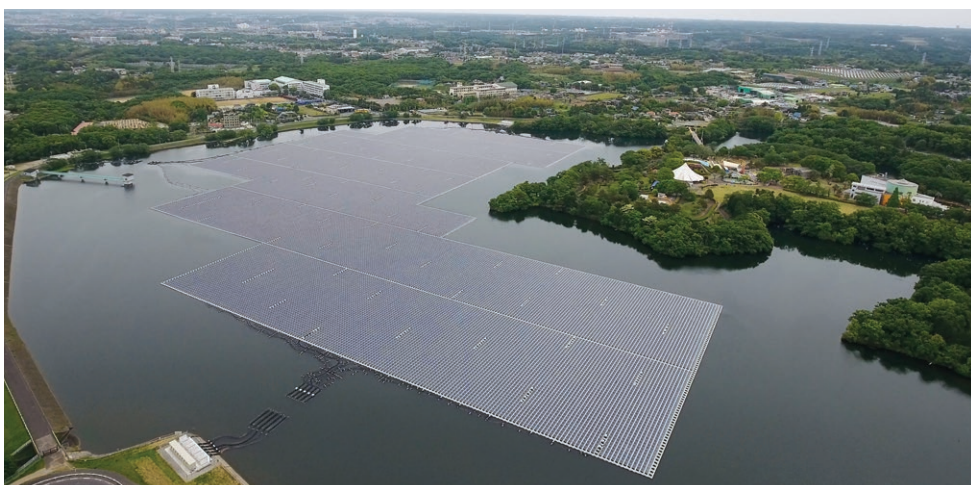
50,000 solar panels create a 1.35 MW floating solar system at the Yamakura Dam in the Chiba Prefecture, just east of Tokyo.
