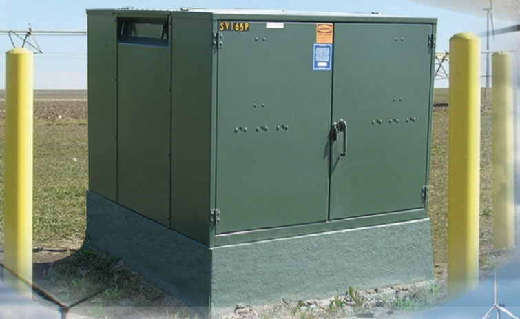
Box Pads for Switchgear
