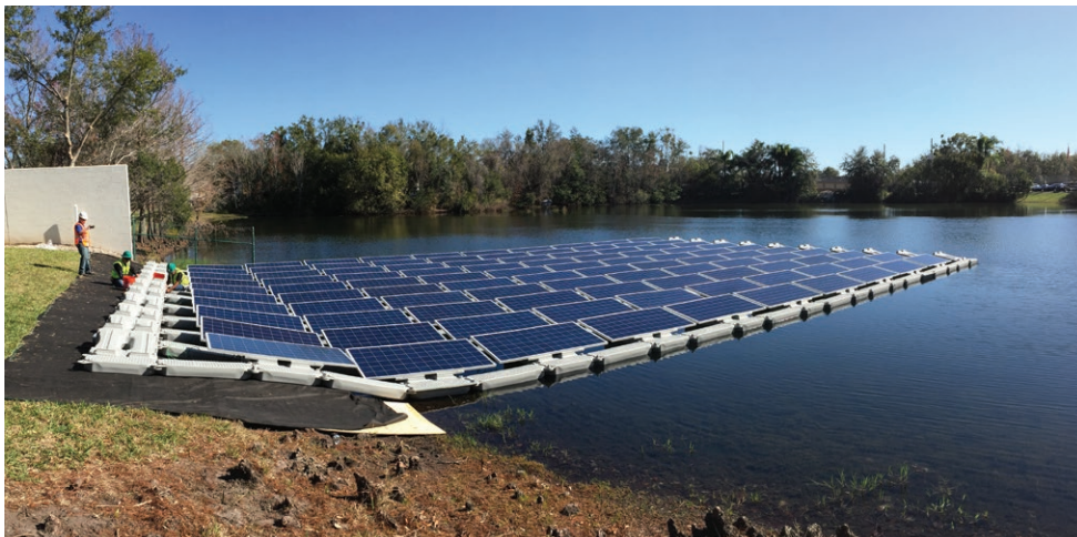
A 31.5 kWp floating solar system at the Orlando Utilities Commission's storm water storage reservoir.
