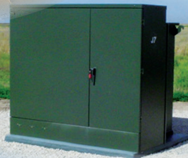
Box Pads for Grounding Transformers
