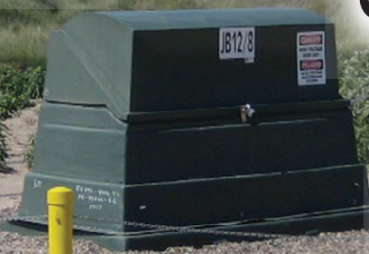
35kV Junction Cabinets
