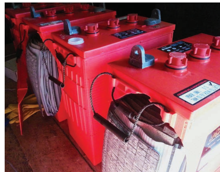
Flooded lead acid batteries which froze due to heavy discharge in freezing temperatures.
