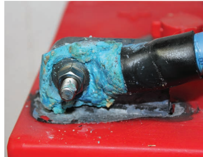
Clean battery terminals and acid spills, and top up cells with distilled water when necessary. Run corrective equalizations when charge imbalance or sulfation/capacity loss is identified.
