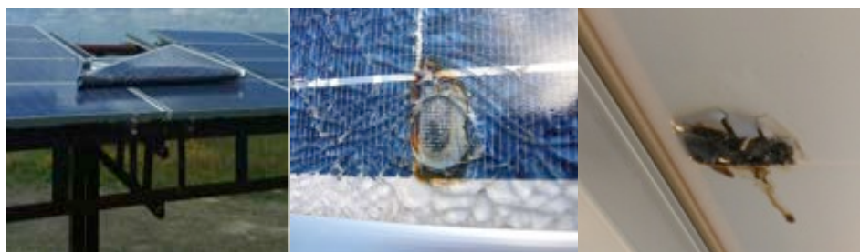
Figure 1. Typical physical DC impairments (from left to right): poor mounting, resulting in module damage, internal short, and damage from falling rock.
