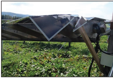
Figure 10: Severe damage due to insufficient embedment depth of the pile foundation
