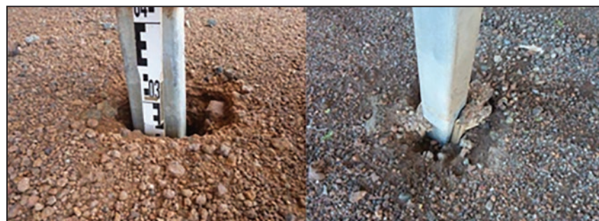
Figure 9: Left hand side: Dynamic loads led to compaction of insufficiently compacted Cut & Fill; right hand side: Subcontractor tried to hide problems he faced during installation
