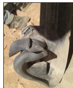
Figure 7: Damaged pile foot due to ramming obstructions
