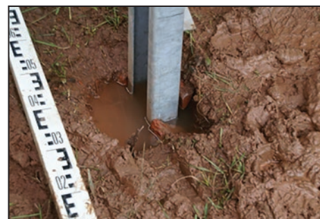
Figure 8: Change of soil consistency due to climatic impacts as a potential reason for pile failure
