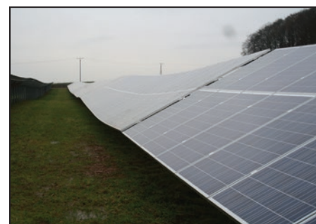
Figure 5: Damage presumably due to Frost Heave
