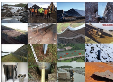
Figure 1: Collage of some structural and geotechnical failures and damages observed at utility scale ground mount solar farms
