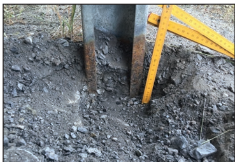
Figure 3: Significant corrosion damage observed at a utility scale ground mount solar farm
