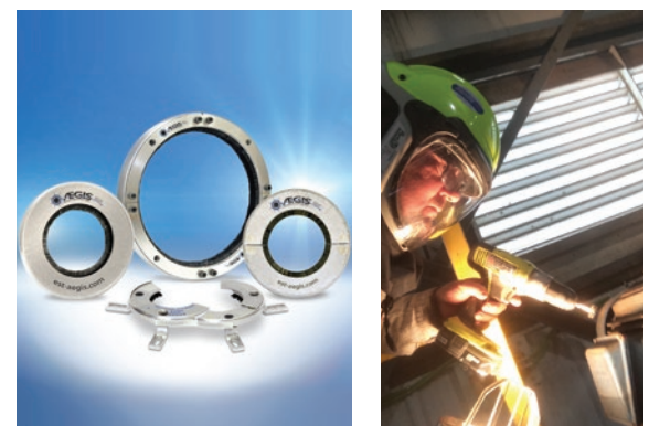
SGRs were installed on the plant's 30 HP and 150 HP centrifuge motors using conductive epoxy.
