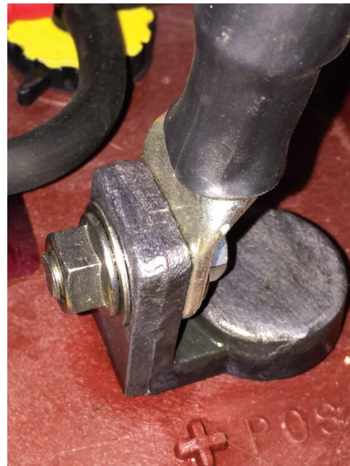
Clean and tighten battery terminal connections for optimum performance
