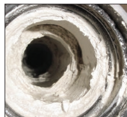
Sulfur deposit accumulation in flow-lines.
