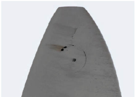
Sometimes lightning damage can be subtle and only high resolution inspection can detect it.
