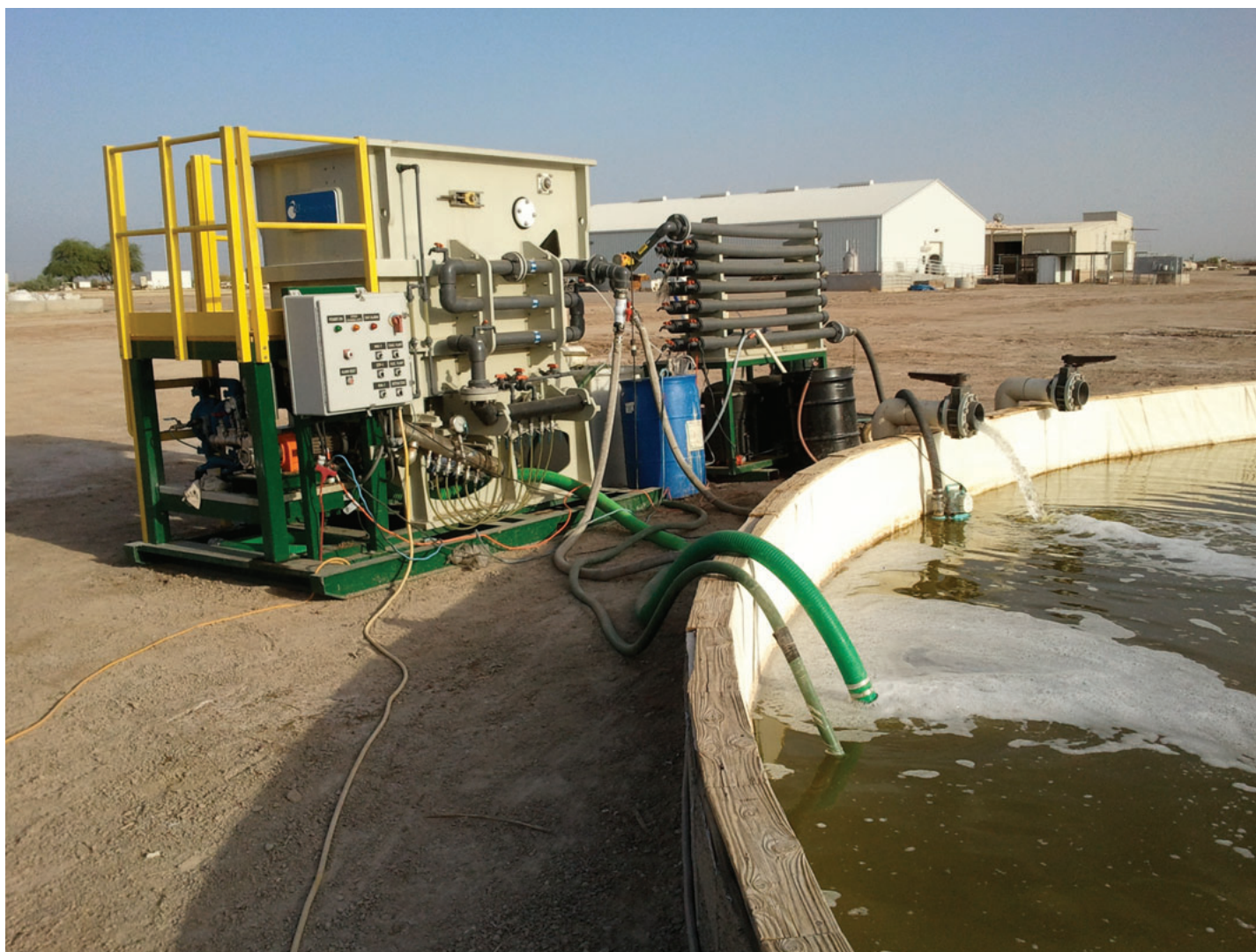
Algae Harvesting Technology Optimized (AHTO) Dissolved Air-flotation system in operation at UC San Diego - Scripps Algae-biodiesel Research Facility in the Sonoran Desert
