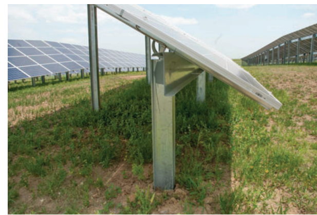
The 500 kW Boulder Cowdery Meadows Solar Array is the first community solar project built under Xcel's Solar*Rewards program
