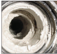
Sulfur deposit accumulation in flow-lines.
