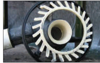
Sulfur fouling on and in the spray nozzles results in uneven water distribution over the fill.
