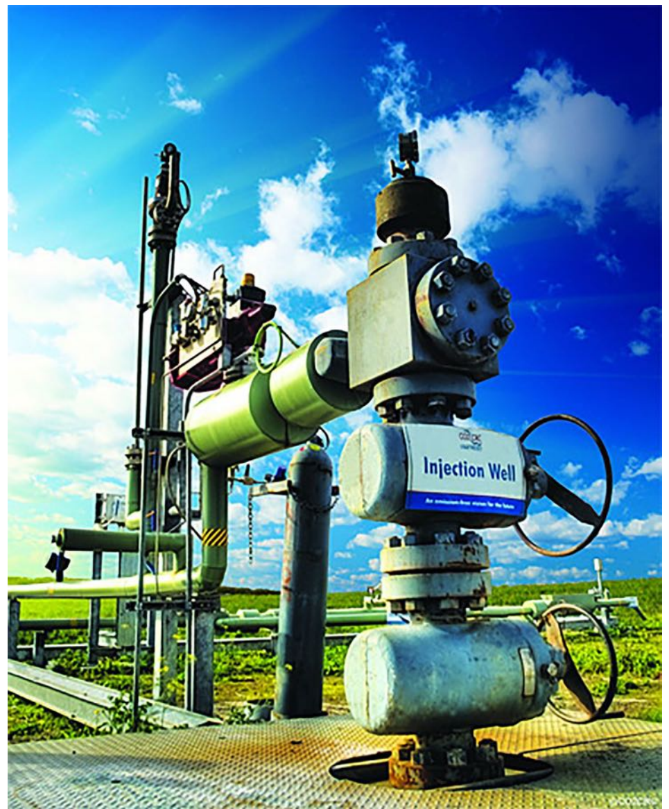
A carbon dioxide injection well (Photo courtesy of CO 2 CRC)
