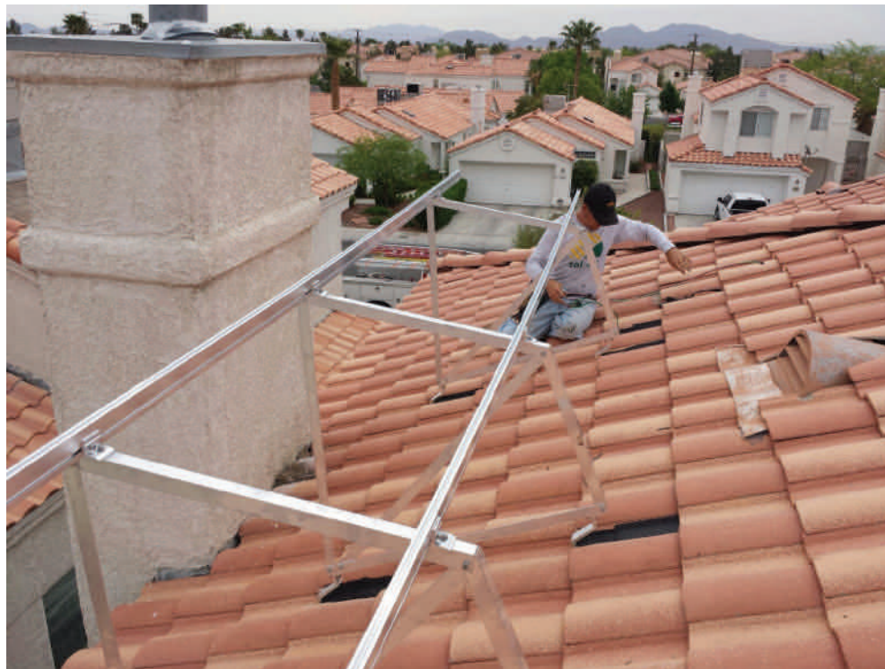
Far Left. Installers at work on a solar rooftop project in Las Vegas Left. Solar “S” profile tiles being installed at a 30-degree angle
